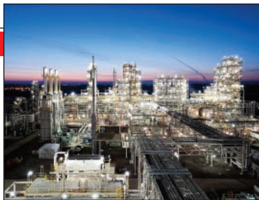
FIGURE 2. Polysilicon production capacity is in the midst of rapid expansion. An example is REC Silicon's facility in Moses Lake, Wash.
