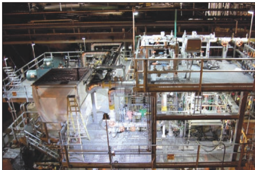
FIGURE 7. As seen in this photo, taken in the field at a gas-recovery unit, the use of new LED-based lighting technologies can lead to tremendous visual acuity improvements at petrochemical facilities by providing adequate light where it is needed the most (throughout the multi-level platform). Notice that the penetration of the light from the higher elevation of the structure down to the lower floor, and the distribution of light throughout the entire structure provides optimum overall illumination
